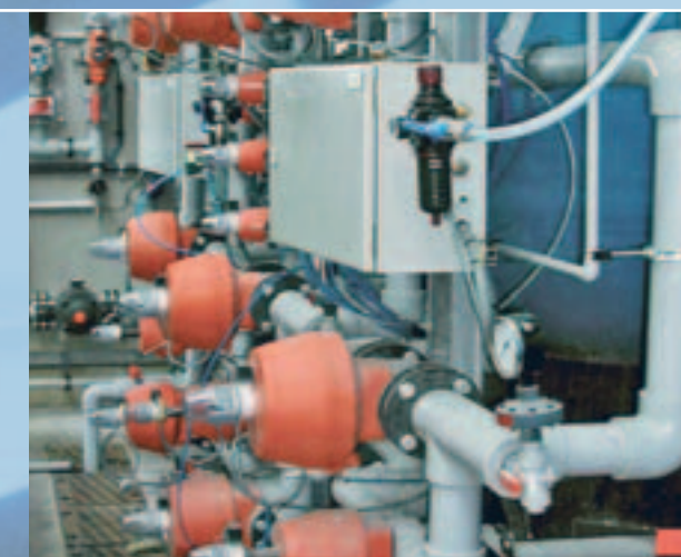
Systems for the chemical stage of a major sewage treatment plant.
