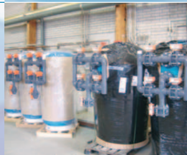
Water Treatment system for Ship Building with PVC-C and PE 100 piping and actuated valves for process control.
