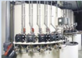
Chemical Injection System
