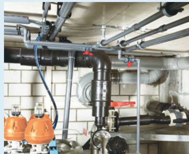
Chemical Conveyance – double containment system
