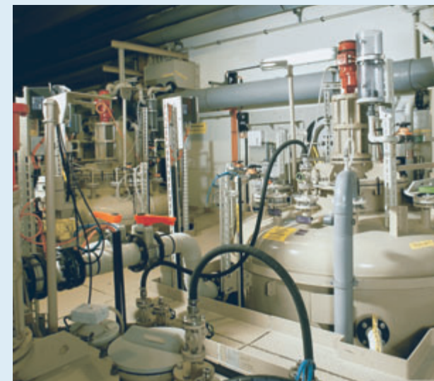
Chemical Drainage and Waste Water Treatment
