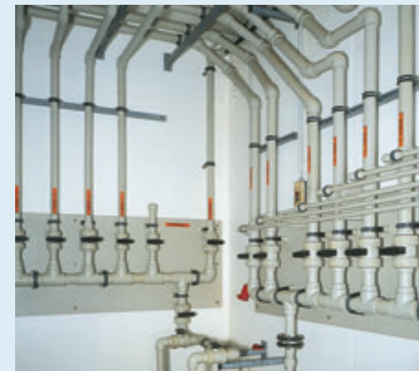
Vacuum system in (β)-PP-H.
