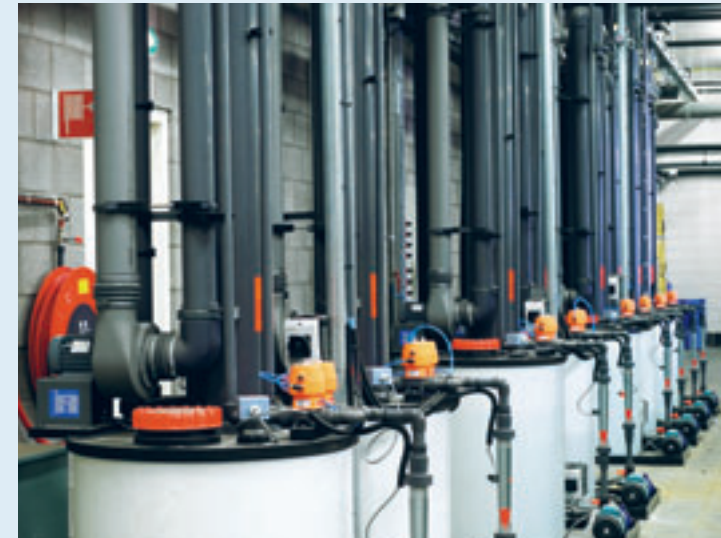
Chemical distribution with PVC-U.
